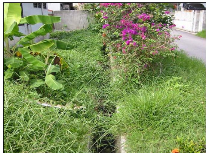
Figure 7. Lack of Maintenance. (MPSP, 2004)
