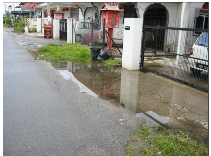
Figure 6. Flooding occurs after a few minutes raining due to roadside drains are not provided. (MPSP, 2004)
