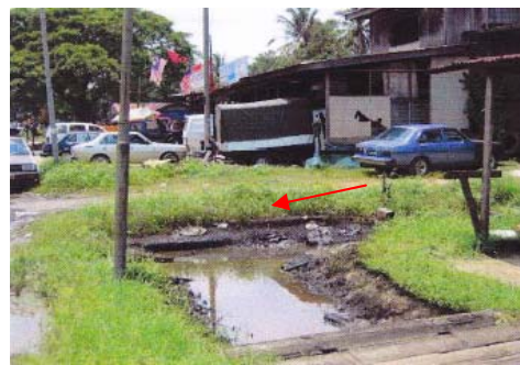
(b) Effluent discharges into main drains
