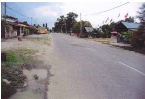
(c) Main roads without main drains
