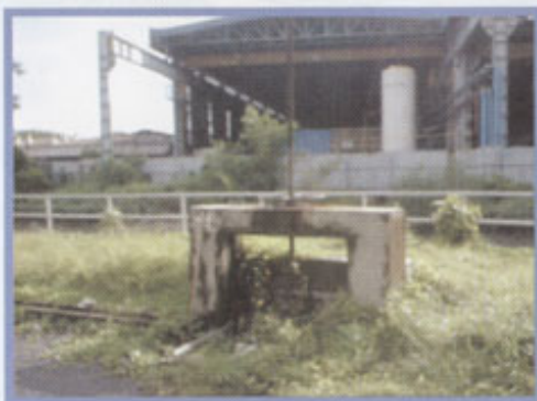
Existing Drainage Condition at Chain Ferry
