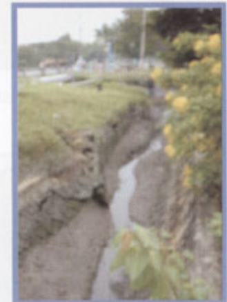
Siltation in the Existing Drain
