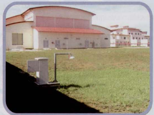
Dry Pond Monitoring Station Site No 2
