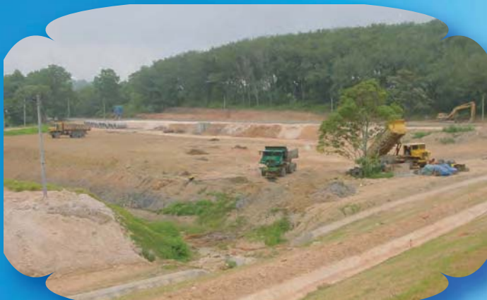
Soil Erosion at Construction Sites
